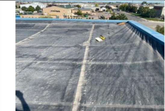
Overview of wind damage
