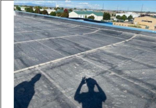
Overview of wind damage
