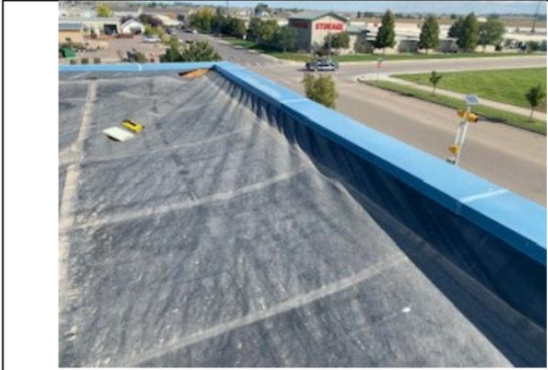
Overview of wind damage
