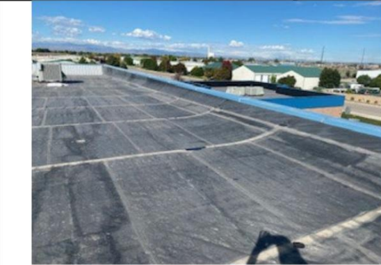
Overview of wind damage
